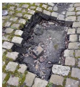
The path had become a health and safety hazard.
